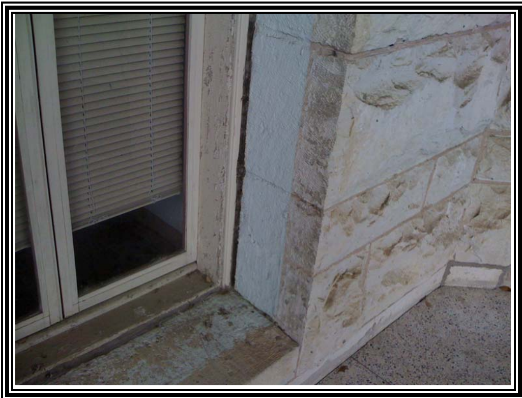
4. View of white LBP on exterior wood window frame.
