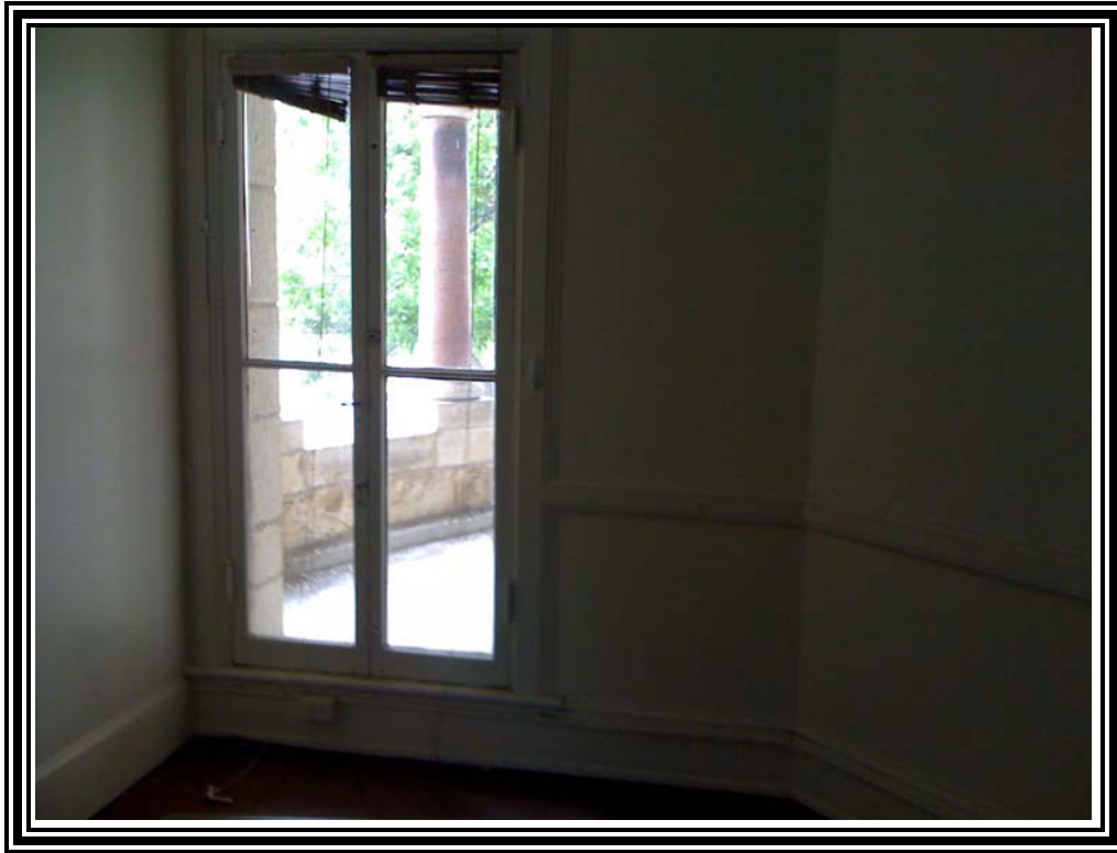
5. View of white LBP trim on the 2 nd floor of the Comal County Courthouse.
