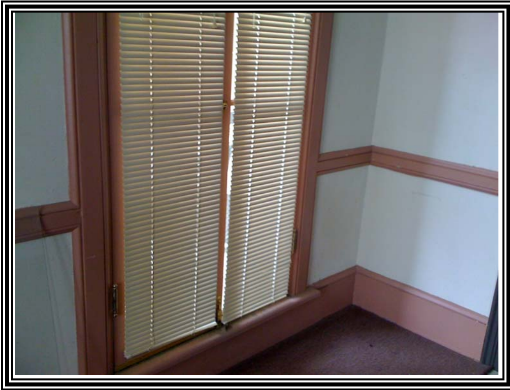
1. View of brown lead-based paint on interior wood window components, trim and baseboards on the first floor of the Comal County Courthouse
