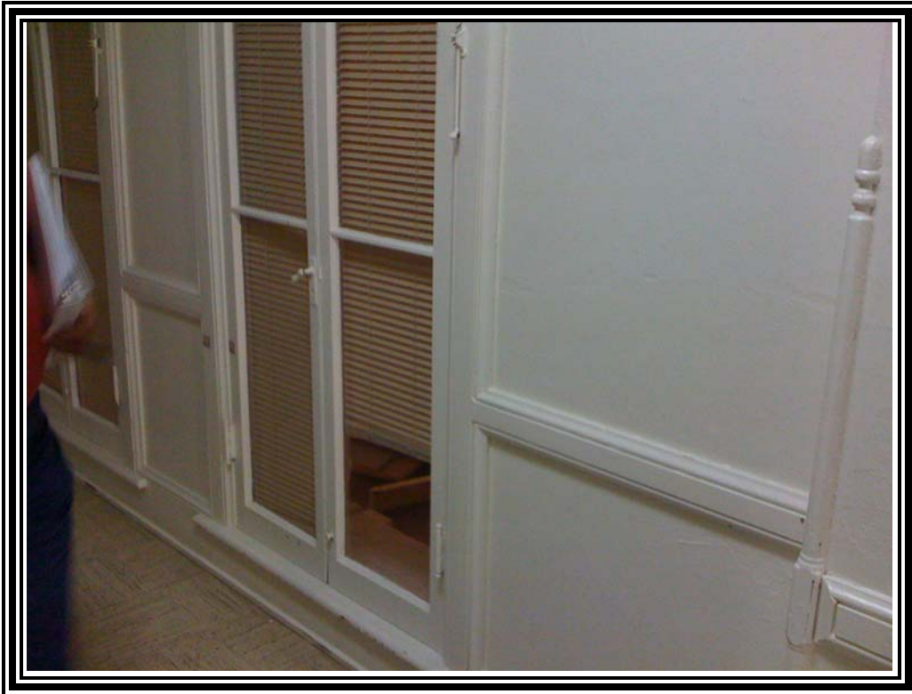
3. View of white LBP on wood trim on the first floor of the Comal County Courthouse.
